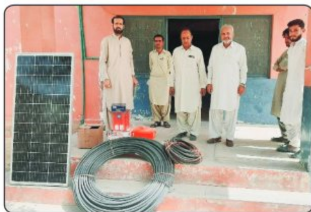
Provision of Solar Panel and Water Pipe Line for BHU Bagbana District Khuzdar
